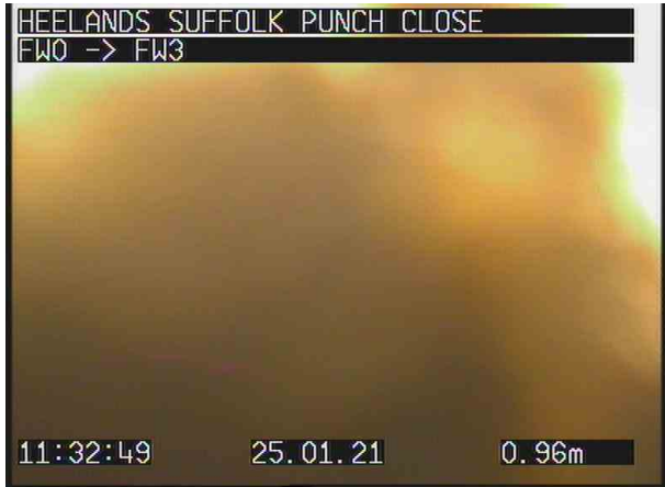
FW0X_2021-01-25 111652_2.jpg, 00:00:18, 0.96 m Settled deposits, fine, 10% cross-sectional area loss, start
